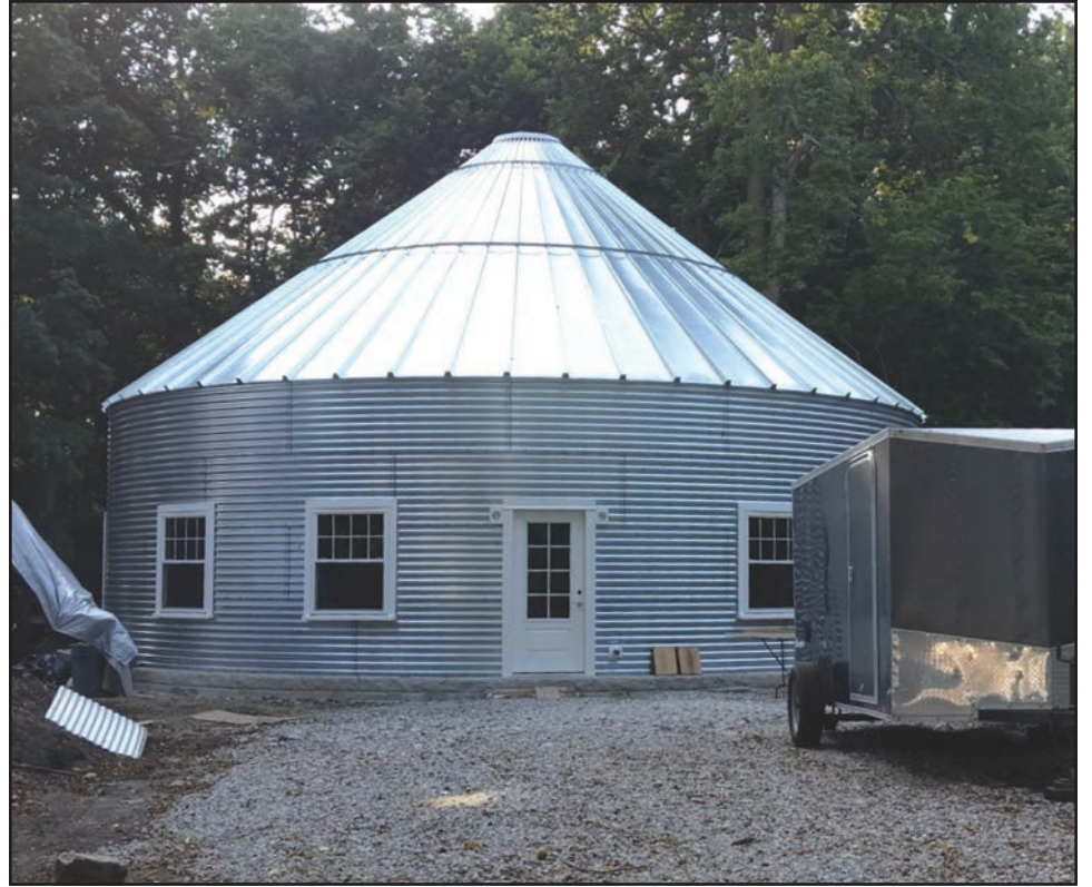
The Island's first silo house is under construction on the west side.
